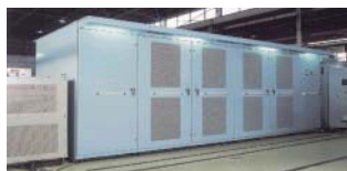
6.6kV Thyristor inverter Control Panel
