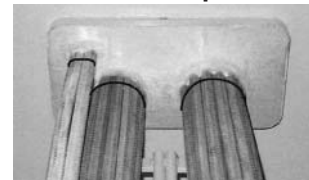
Consider the size of any additional cables to be used by cutting the thermal foam blocks, and packing the space with the cut-off pieces of the blocks after laying the cable.
