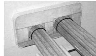
Pack the space around the cable in the coaming with thermal foam blocks (gaps of about 5 mm will not pose a problem).
