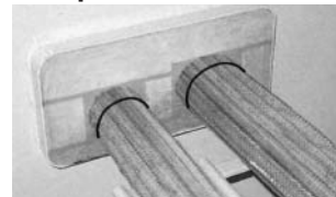
Fill block seams and the space around the cable with silicon to prevent the small thermal foam blocks from falling. The installation is now complete.
