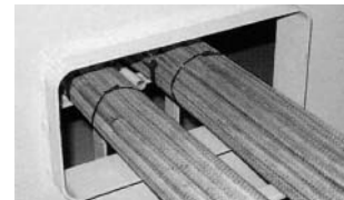
After putting cables together to between 150 and 200 Ø, fix it in place with binding lines or winding belts.
