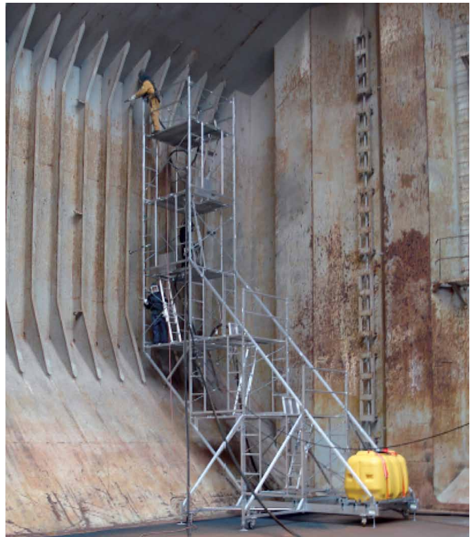
Maintenance Staging Tower for bulker hold.
