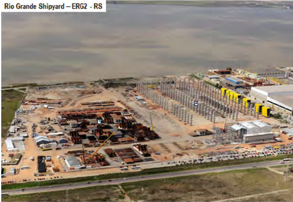
Works' Aerial View of Estaleiro RioGrande2 (ERG2) – RB (0803/12). Construction work of the Estaleiro ERG 2 where it will be built 8 Setebrasils' Vessels (NS Cassino, NS Curumim and NS Salinas). (1) Hull's blocks of SFRBOs replicating (P-05, P-07, P-08, P-09, P-10, P-11, P-12, P-13), which it will mount in the ERG1 by Ecovix; (2) ERG2's workshops civil construction
