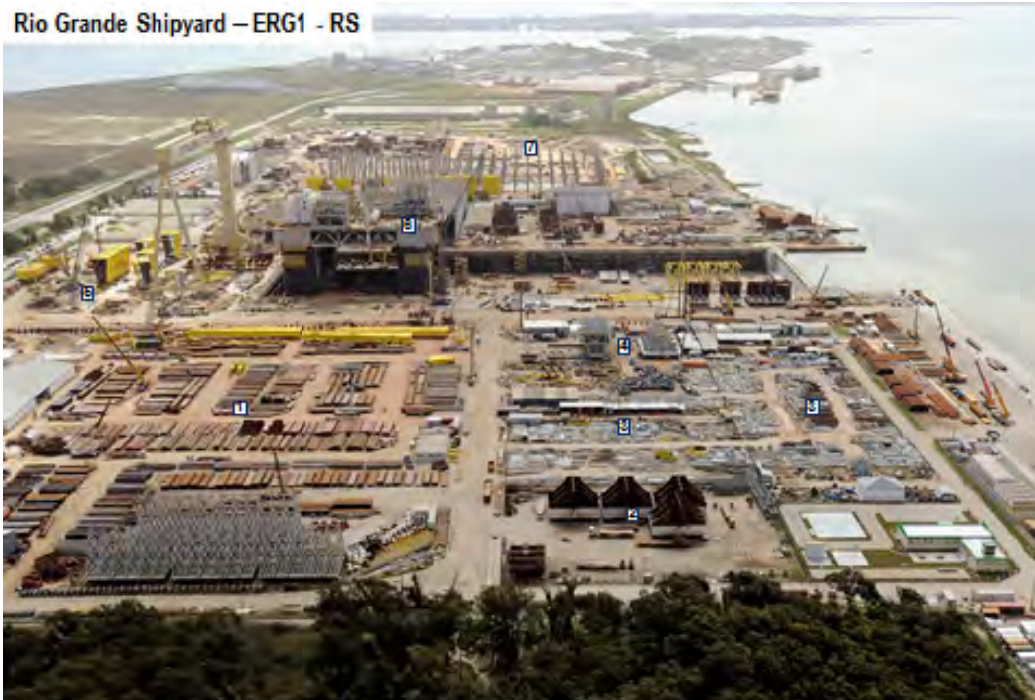
Aerial View of the Estaleiro Rio Grande ERG1 - RS (09/03/12). (1) Ecovik's Sheets Yard, (2) Sub-blocks Yard of Ecovik's replicating hooves, (3) QUP's modules gantry for topside and integration of the P-55, (4) IESA's modules gantry, (5) Re-construction area, with detail to the yellow blocks of Konecranes' Goliath type portico (largest crane in the world, 210m span and capacity of 2,000 tons) delivered in Aug/12, (6) integration work of the P-55, (7) Construction work of Estaleiro ERG2, where it will be built 3 Sotobest's Driships (NS Cassino, NS Curumim and NS Salinas)
