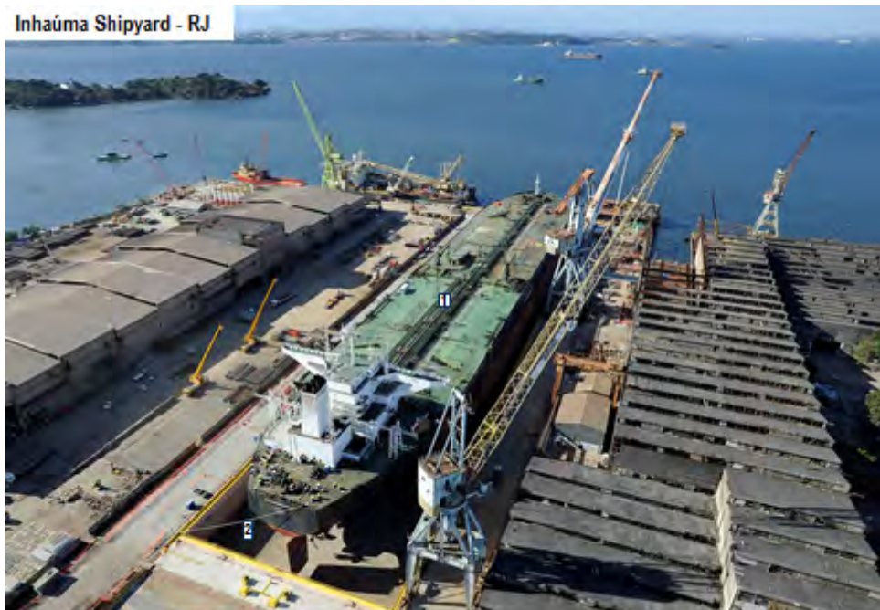
Overview of Estaleiro Inhaúma, in Rio de Janeiro - RJ (08/61/12). (1) P-74: Conversion of the ship VLCC's hull (hull structural reinforcement, expansion, renovation and adaptation of accommodation, equipment installation and anchoring system's adjustment and utilities). (2) Dry dock recovered by Petrosas.
