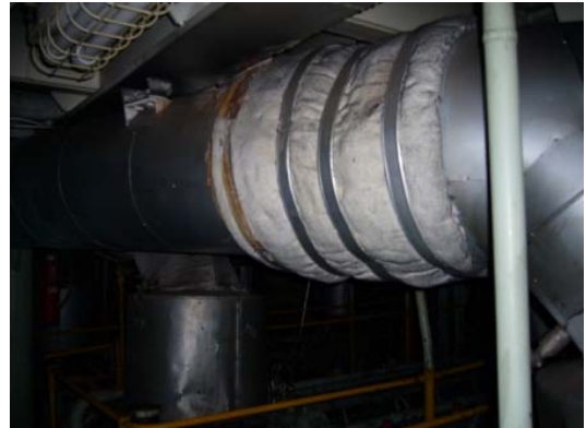
(Asbestos blanket on expansion section of exhaust pipe)
