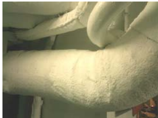
(Asbestos cloth wrapped around steam pipe)
