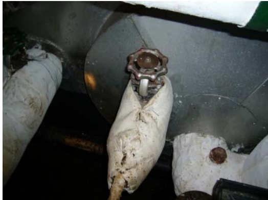
(Asbestos blanket used on steam valve)
