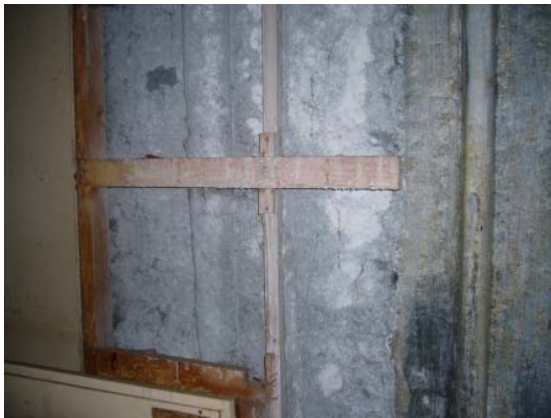
(Sprayed-on asbestos on reverse side of wall in accommodation space)
