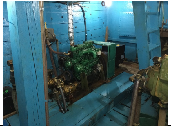
前頁漁船の発電機 (Marelli Motori, Made in Malaysia)
