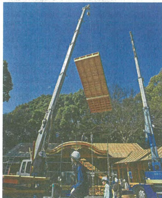
The hinoki cypress stage is disassembled at Meiji Jingu shrine on March 13. It was to be transported to a warehouse in Nara Prefecture.
