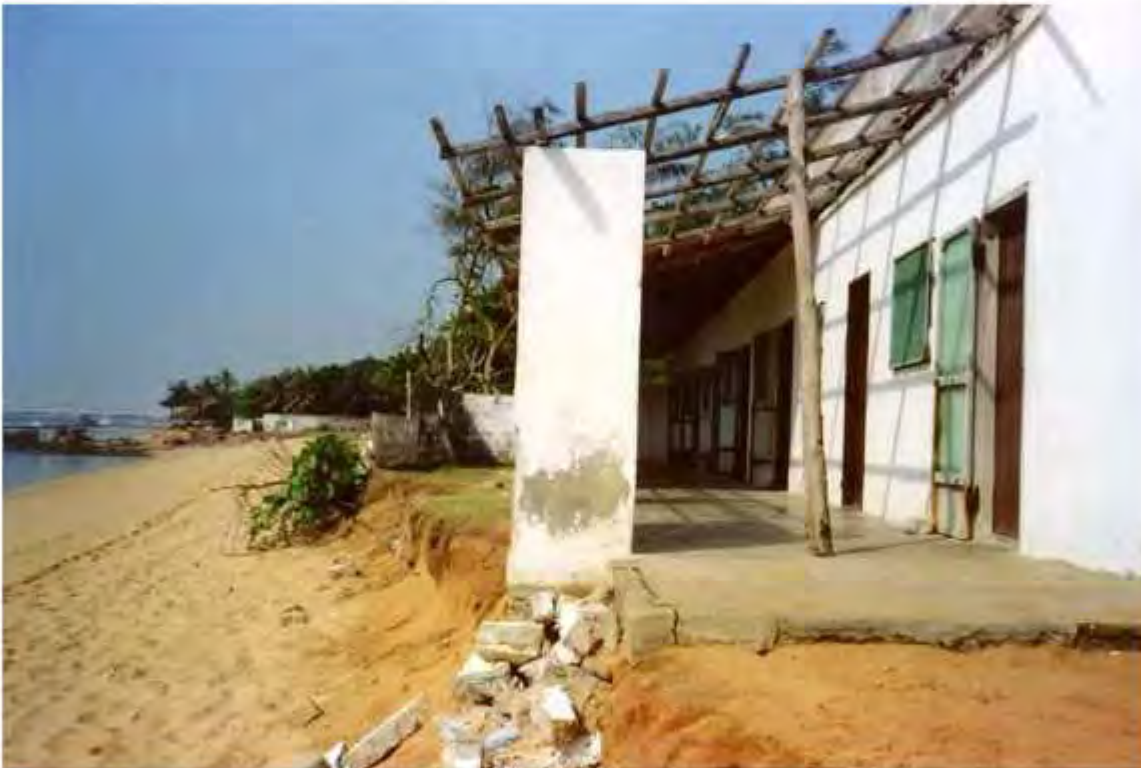
Figure 4: Beach affected by coastal erosion at the Ramatou Hotel (east of PAL) in November 2003
