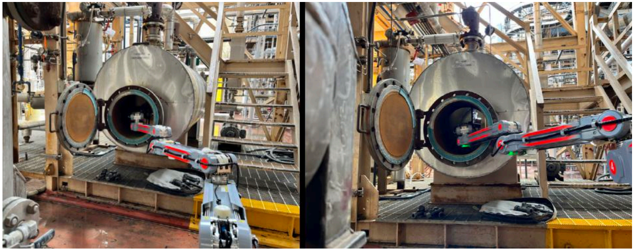
The arm is inserted in the vessel tank while avoiding the vertical internals standing in front of the manway
