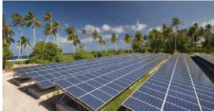
PV installation, Nukunonu atoll, Tokelau
